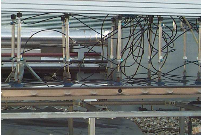
Figure 4: Negative pressure test of fixings between the cover and the collector box
